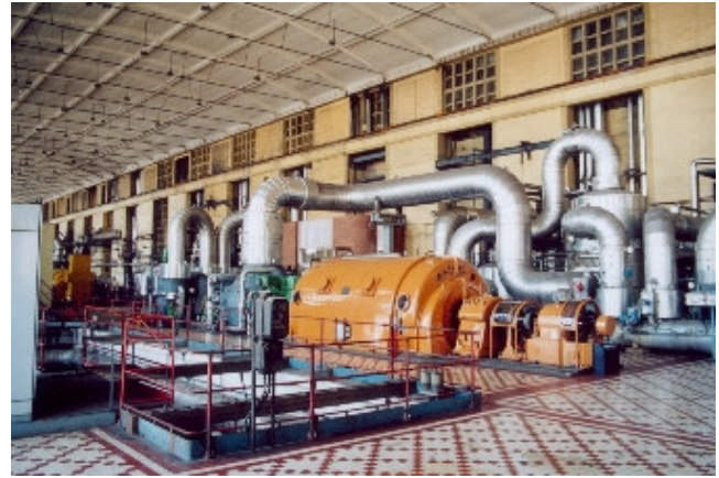
Fig. 6.: A 40 years old 30 MW heat-coupled unit at Pécs power plant
